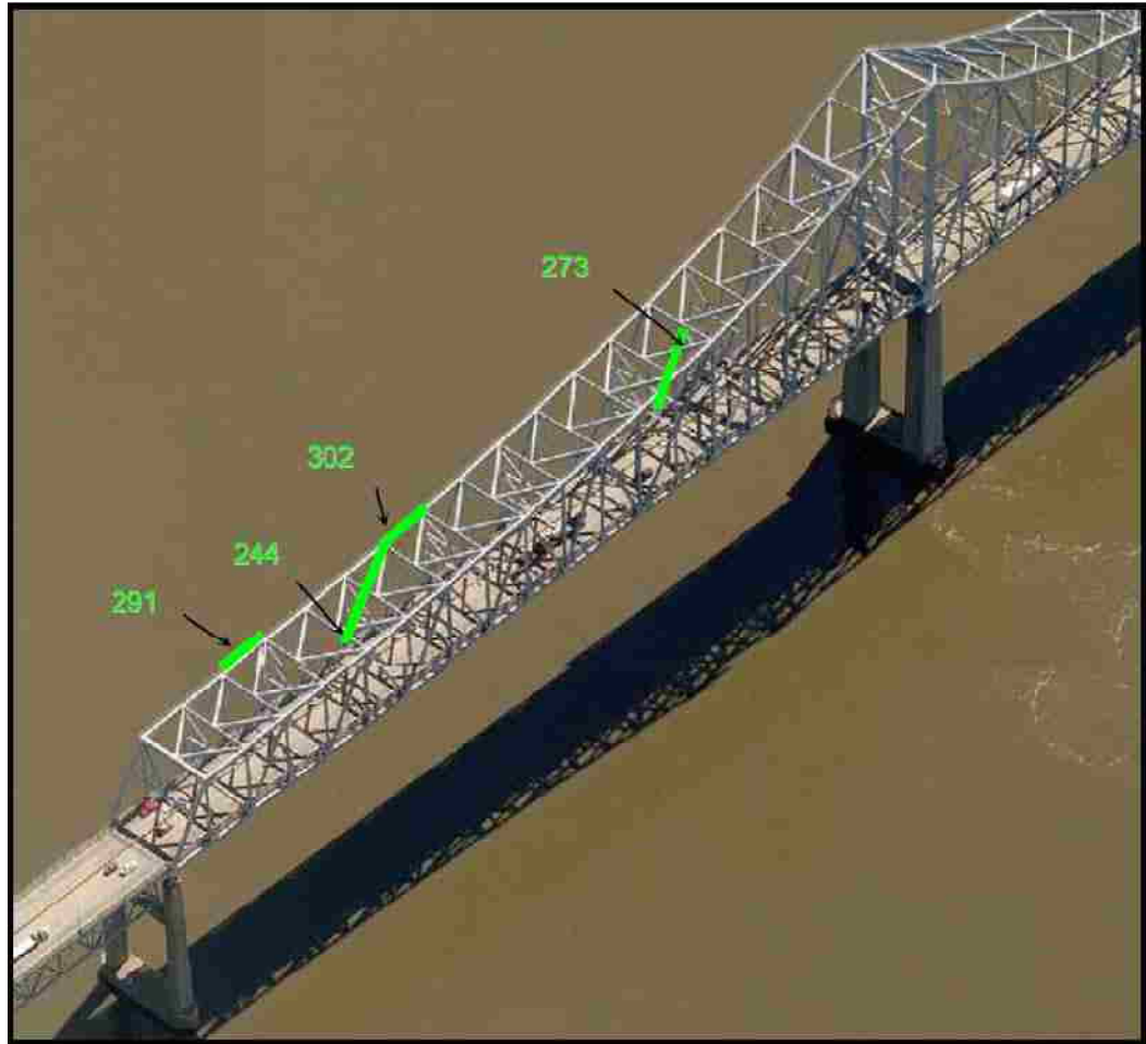
Figure 5.3 Photographic view of Pennsylvania back span looking upstream showing instrumented truss members (green = upstream; yellow = downstream) (From Hodgson et. al, 2008)
